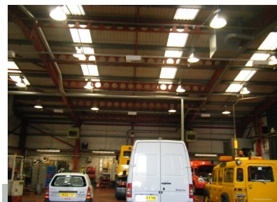
Motor transport area has improved light levels to 850 LUX from 350 LUX previously. Power consumption has been reduced by two thirds.
